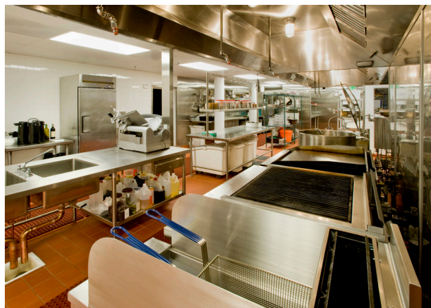
This photo illustrates the correct installation of a metal baffle plate between the open flames from the range and the deep fat fryer. Metal baffles should be used only when there is not sufficient space available to provide a 16" clearance between the deep fat fryer and any source of open flames. Baffle filters are seen above the range and fryer.
